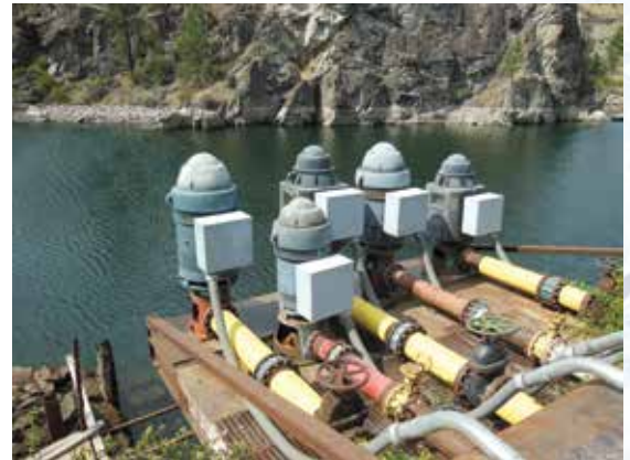
Quadplex River Booster System.
