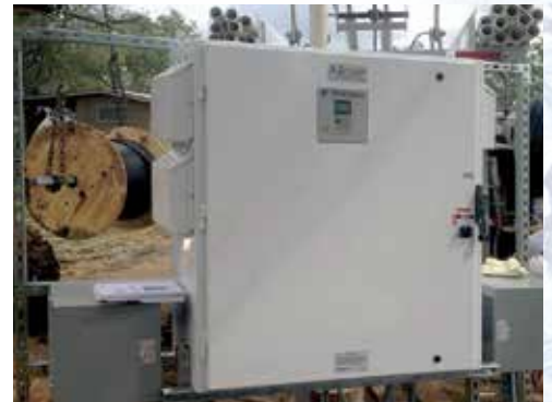
20 HP Submersible Pump Control for Irrigation.
